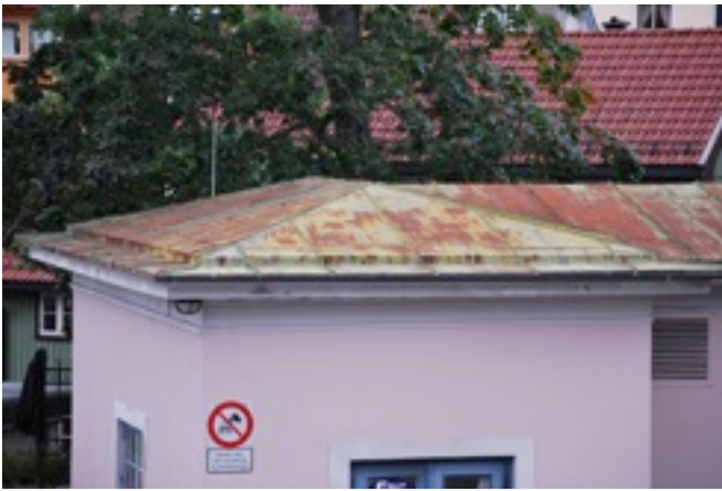
Drosjebu, trafokiosk, v/ Drøbak torg.
