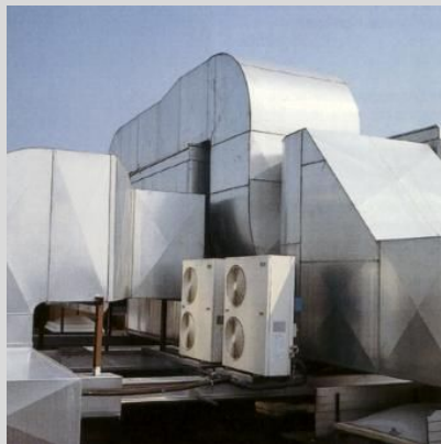
air conditioning ducts on roof
