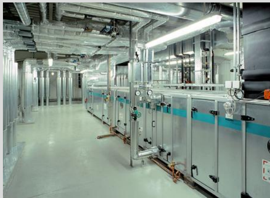
air conditioning system
